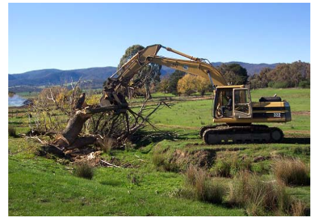
Willow control works on John Pennington property May 2003 this area will be fence and revegetated
