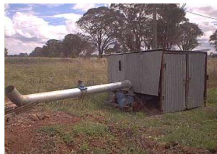
Flow meter on pump discharge line
