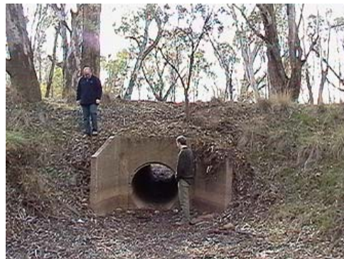
This culvert was a barrier to fish movement into Horseshoe Lagoon near Cobram, and has been removed.
