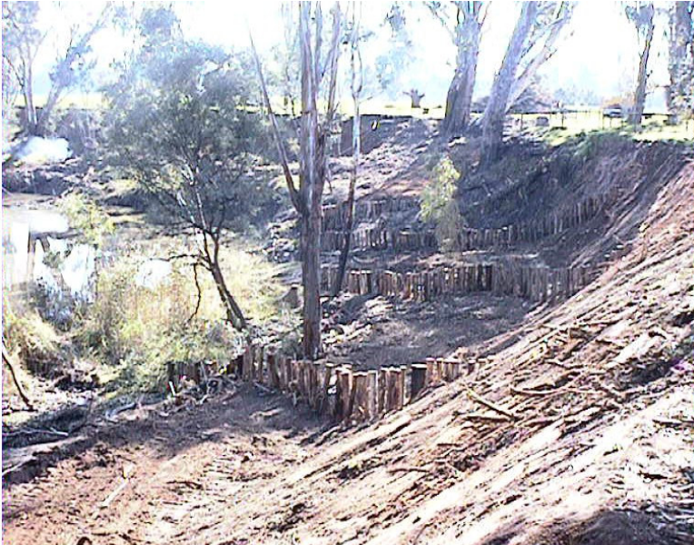
Photograph: Woody weed removal and bank stabilisation works on the Goulburn River
