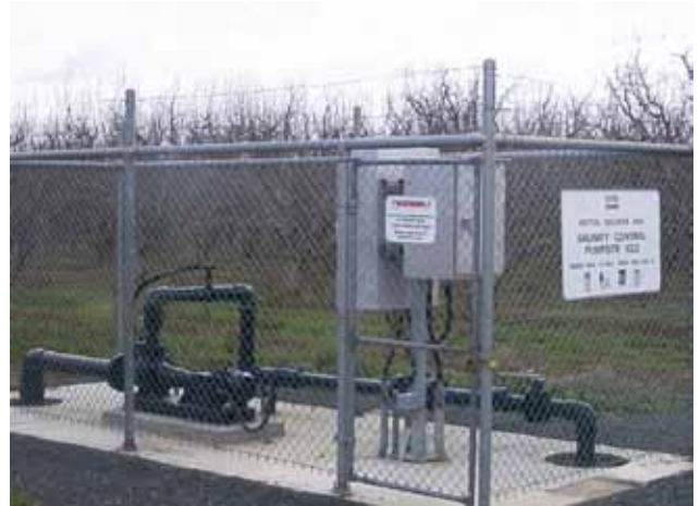
A salinity control pumpsite
