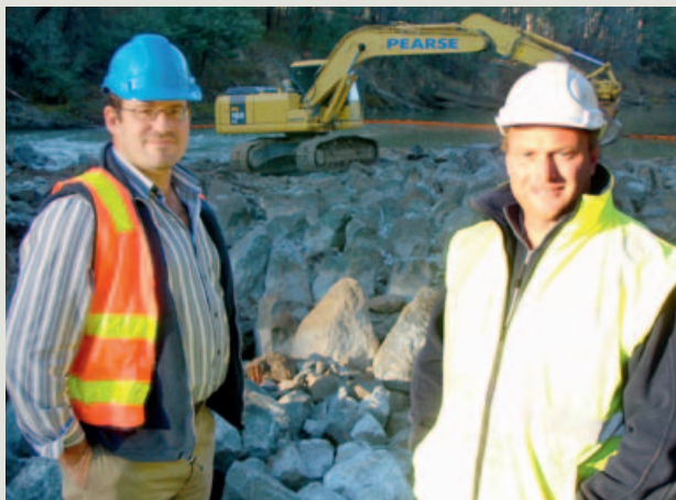
GB CMA's Carl Walters and Corey Wilson inspect works on the Goulburn River. Photo: Mark Turner, GB CMA
