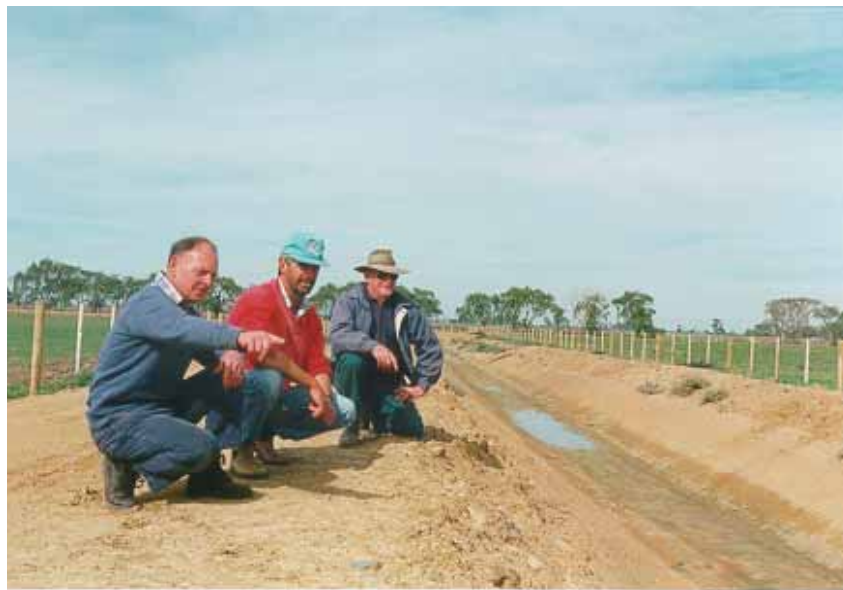
Figure 2 – Rodney 1/6P Community Surface Water Management System, Completed 1995, Stan Nixon, John Poppa, and Jim Kay
