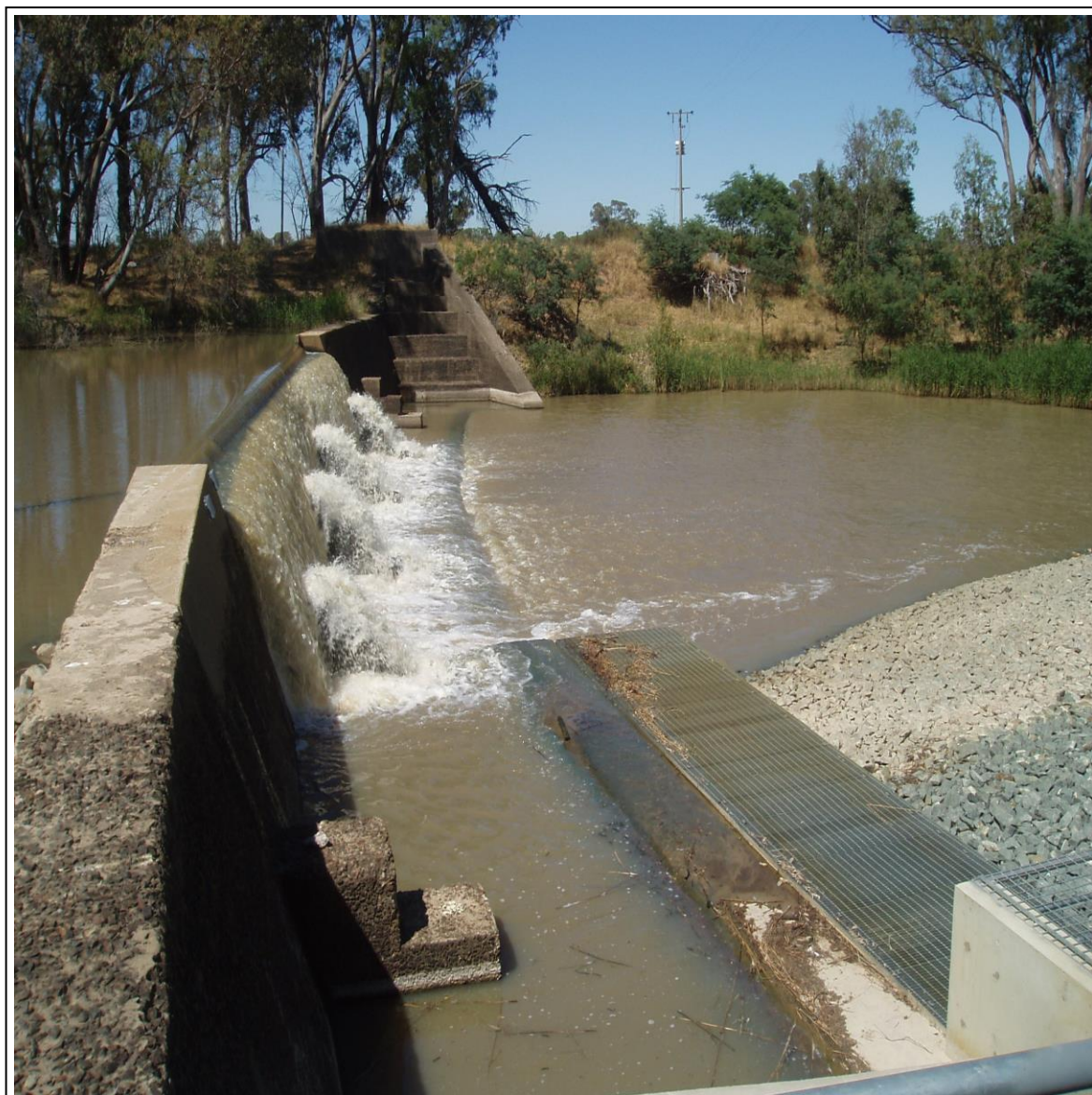
Figure 33 Fish ladder on Broken River, at Casey's Weir
