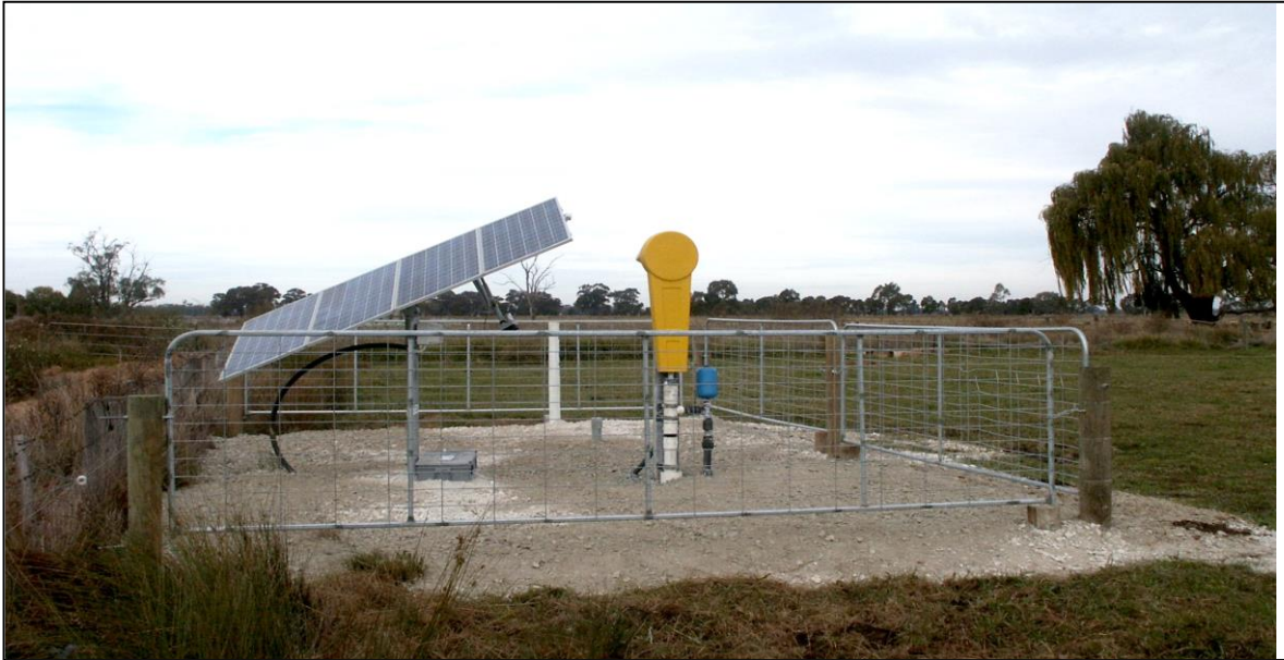
Figure 31 Solar powered low volume pump near Wyuna
