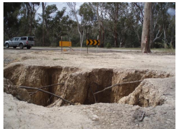
Tunnel erosion site on Murray River Echuca
