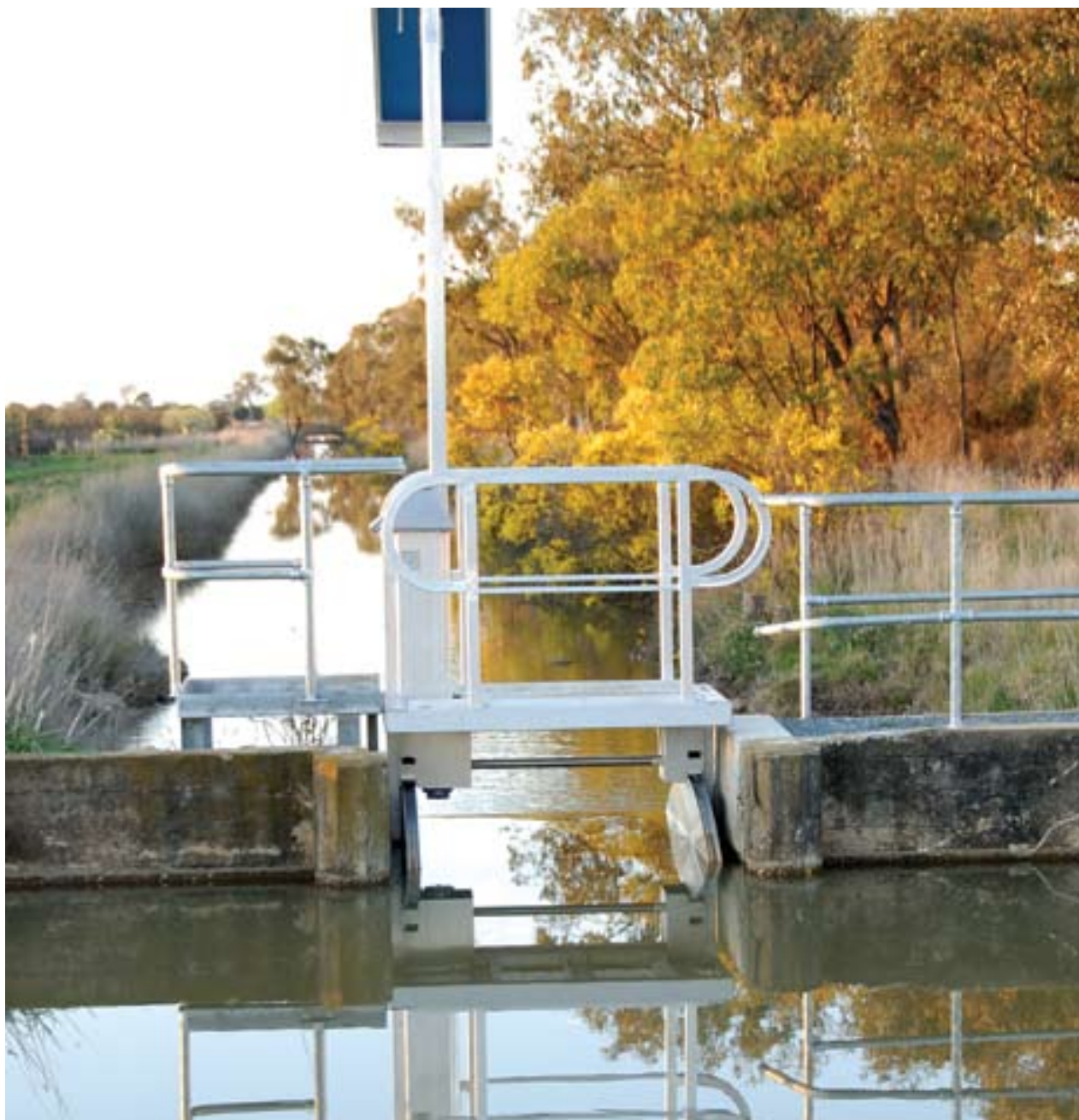
Automatic irrigation channel gate
